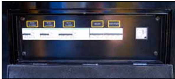
RCD protection for all high voltage circuits
